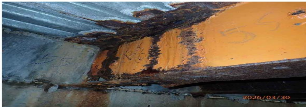
Photo 6: Beam 5, South Abutment, East Face - Web and bottom flange section loss and holes in web at support
